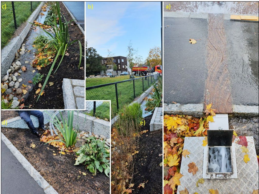
Figure 6. Photographic documentation of the 23 October 2023 stress test showing inflow at Inlet 1 (a), mid-section flow conveyance (b), approaching flow near the outlet (c) and discharge into the downstream manhole (d).
