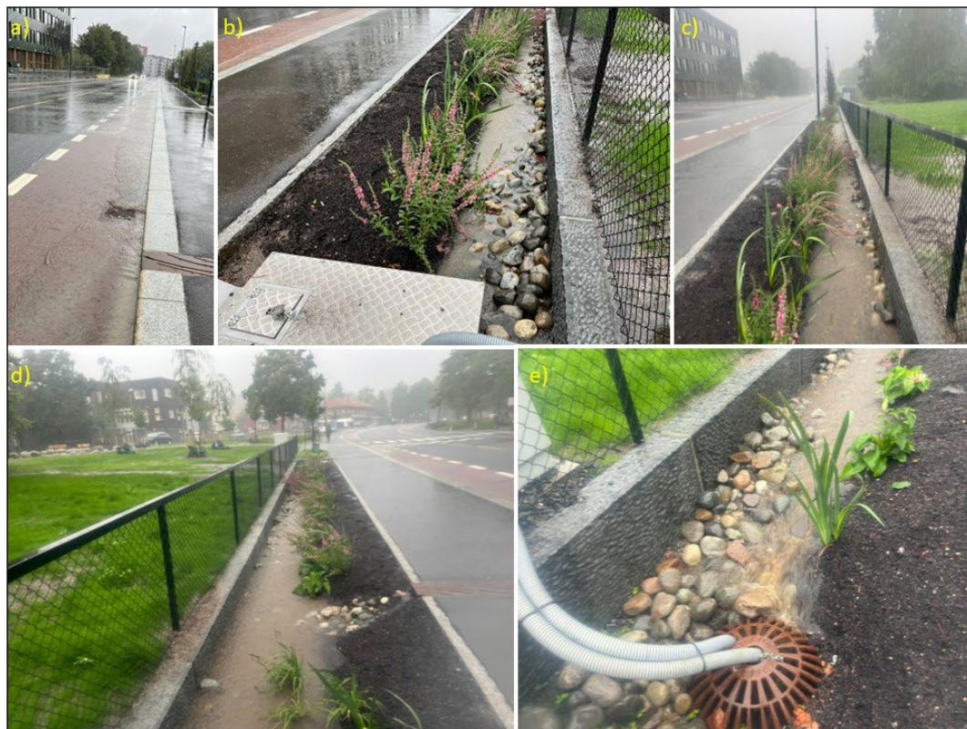
Figure 3. Observed hydraulic behavior of the roadside NbS facility during an intense rainfall event associated with Storm Hans (07 August 2023, afternoon). (a) Runoff from the road surface and bicycle lane entering the system; (b) Inlet zone showing ponding and additional inflow from the adjacent lawn; (c) Mid-section illustrating conveyance of runoff along the trench with continued lateral inflow; (d) Downstream section showing temporary storage and flow routing within the system; (e) Outlet structure where runoff is discharged to the downstream manhole.
