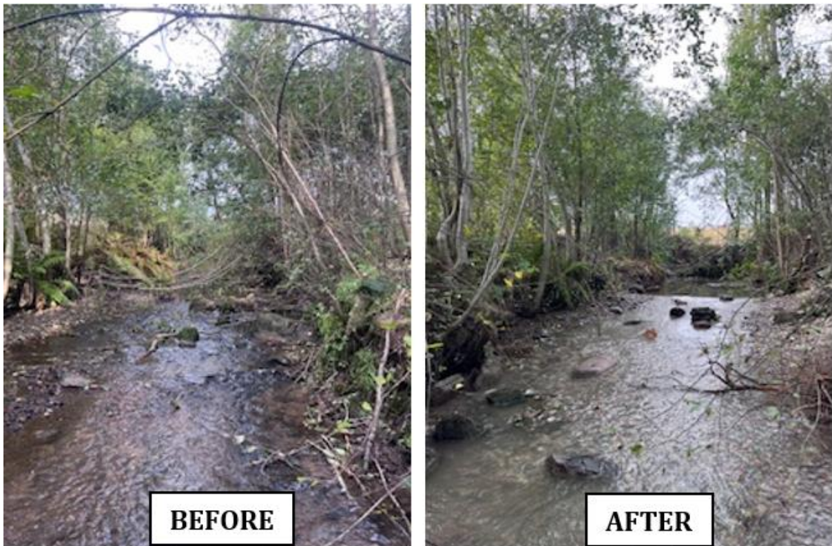
Figure 28. Before and after images of Site 3 restoration, which included full optimization measures.
