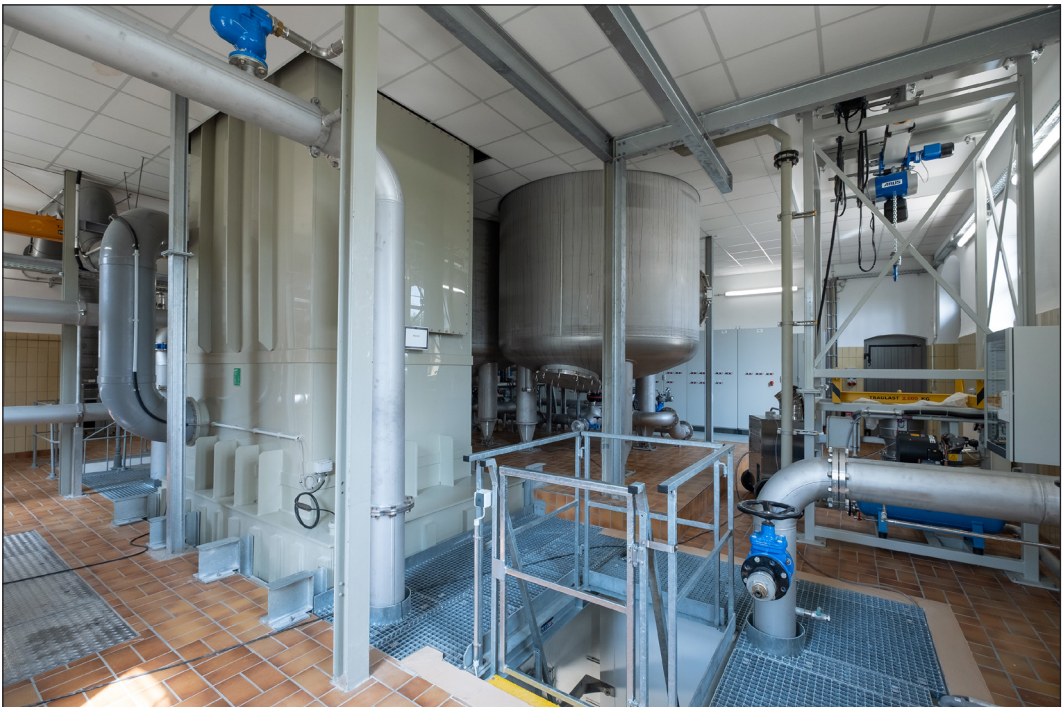
Figure 3. Waterworks for PFAS treatment: Remediation of PMT/vPvM substances is extremely difficult. Source: Marcel Riegel, DVGW-TZW
